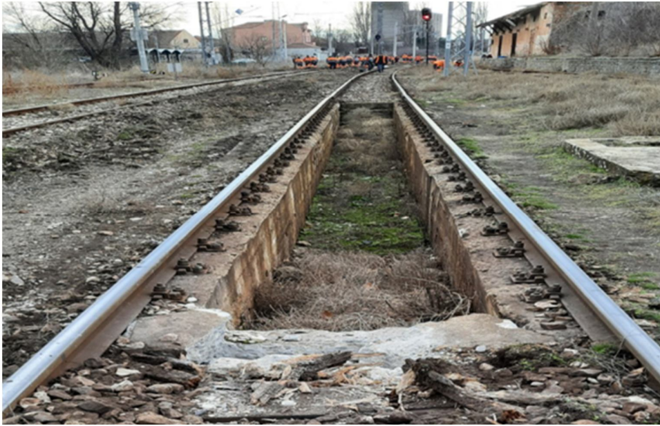
Fig. 3.6. Technological canal on second track in Radnevo station
